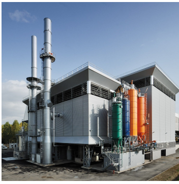
- IT_0039 - POGGIBONSI INCINERATION PLANT - SIENAMBIENTE - 68,312 tonnes. 9.9MWe, 35MWt
